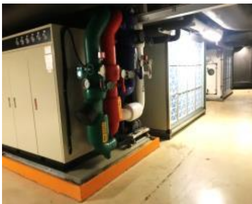
Replacement of make-up air units (traditional heaters replaced with energy-saving heat pumps)
