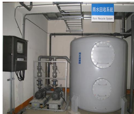
↑ Factories installed with
